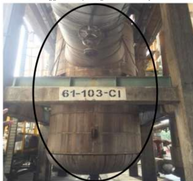
Gambar 1. Heat Exchanger Item 61-103-C1
